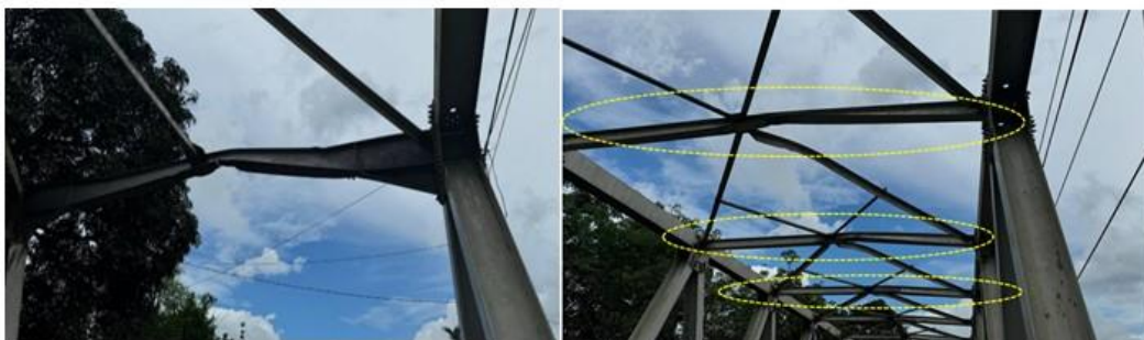
Figure 2. Damaged elements after a crash.
