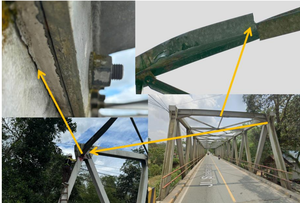
Figure 8(b). Field damage conditions.
